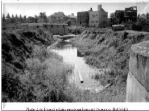
Fig No: 7 Encroached Drainages in Bangalore BBMP
