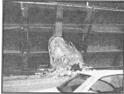
(b) Column separation due to tension generated in longitudinal reinforcement on overturning
